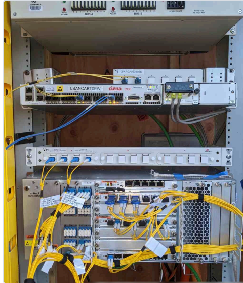
After. Fujitsu HSN8300NA installed under the Ciena 3930 and DC fuse panel; fiber dressed and bundled.
